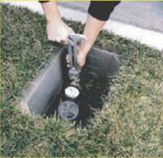
Shuts Off Water
